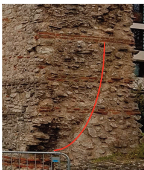
TOP: Roman Wall and core (arrowed in red) with the later repair without tile courses (in black)
